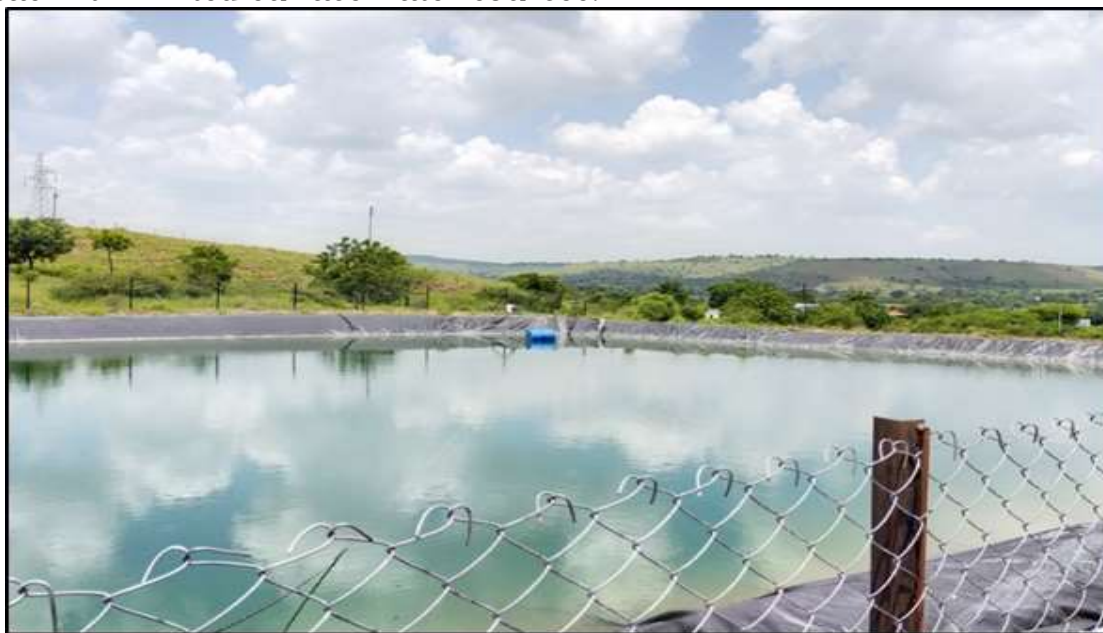
Figure No. 2: Farm pond with Poly-ethane (PE) lining and Galvanized Iron chain link fencing
